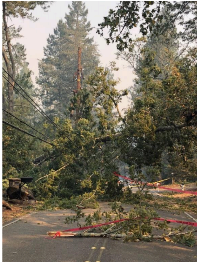
25 A fallen tree blown onto a de-energized PG&E distribution line (Public Safety 26 Power Shutoff Oct. 26–Nov. 1, 2019 Report, Appx. C, Fig. 6).
